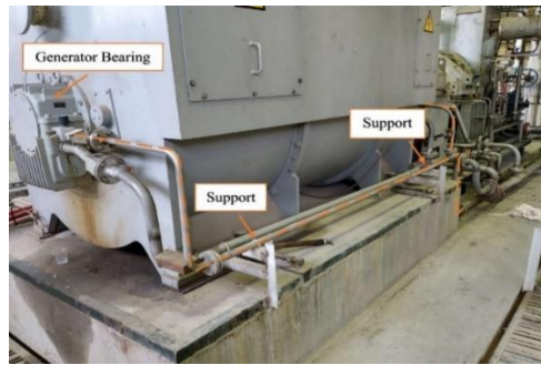
Figure 1. Lube oil piping configuration
